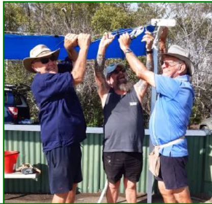
6 February: New Shade installation led by Errol Fender, with Jim Warwick, Ray Black & Rod Curtis
